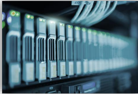
Server & Data Storage
